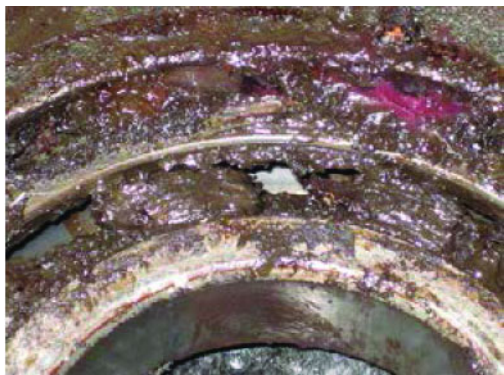
Grease Contaminated With Debris
